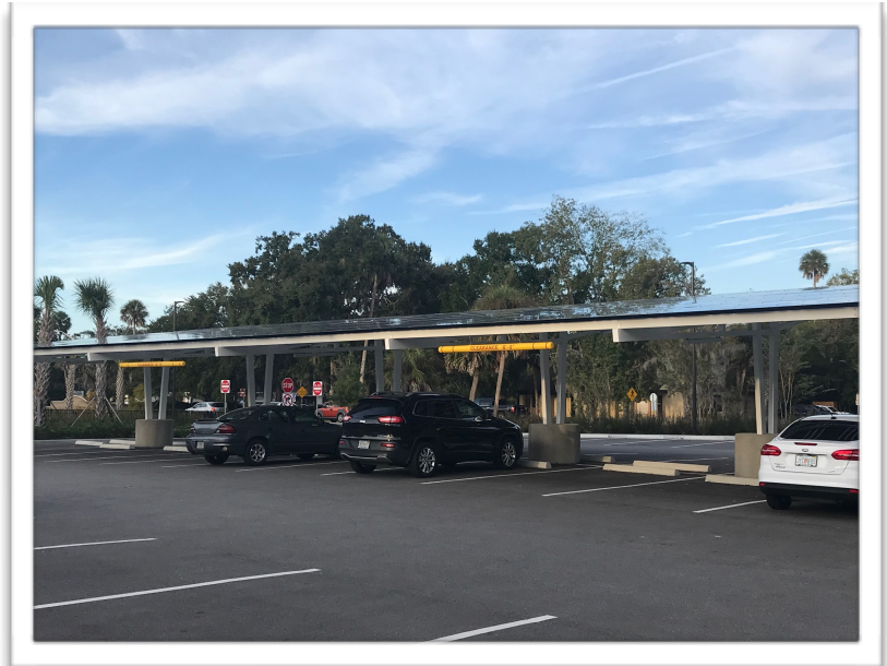
Solar Parking. Palm Coast, FL Community Center
